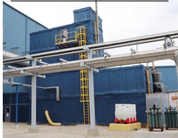
Molten Salt Purification Plant Elmore, OH
